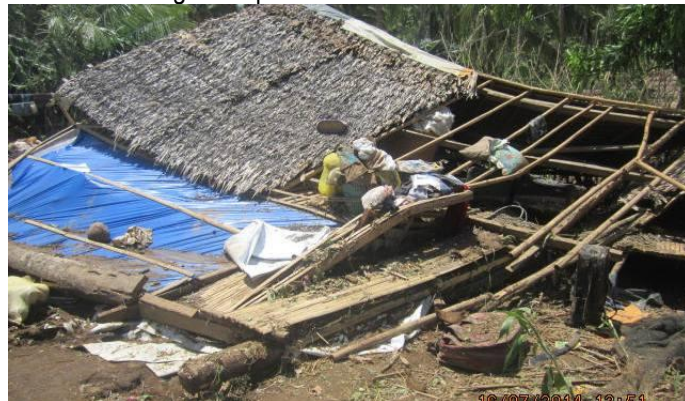
PAMI Bulabog church member Sis Nova's house collapsed.
