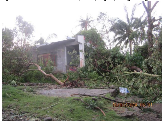
The EBI church roof was damaged, and many trees blown down.
