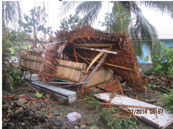
This EBI cottage collapsed & the other one needs a new roof.
