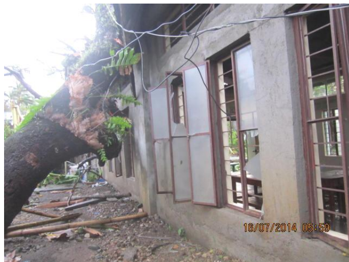
Broken window glass on back side of session hall.
